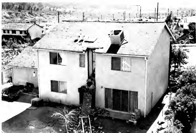
Photo 11. Newly completed structure with repairable damage. Here lateral support was sufficient to prevent collapse. Nevertheless, the chimney fell, windows shattered, and some walls were damaged. Photo courtesy of the City of Los Angeles Department of Building and Safety.
